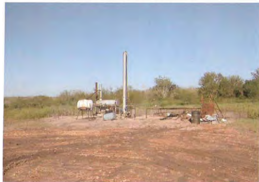
Photo No. 3 – Patrick Welder Tank Battery
